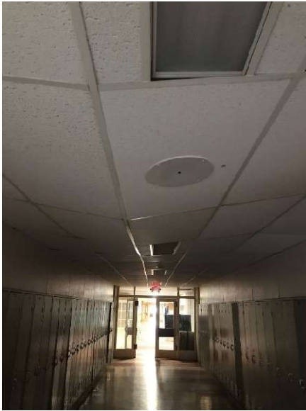
Fig.93 – Damaged ceiling tiles
