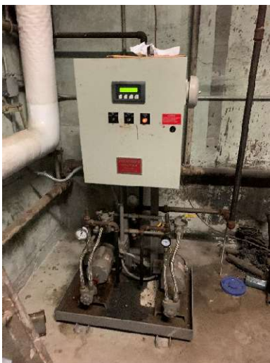
Fig. 9 – Fuel oil transfer pumps
