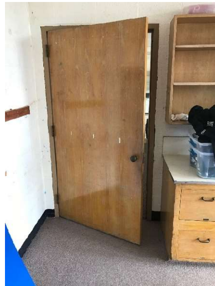
Fig.26 – No ADA front approach clearances
