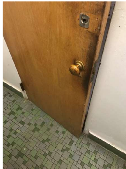
Fig.76 – Worn door & hardware
