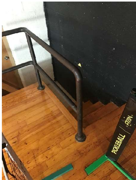
Fig.44 – No ADA handrails at stairs
