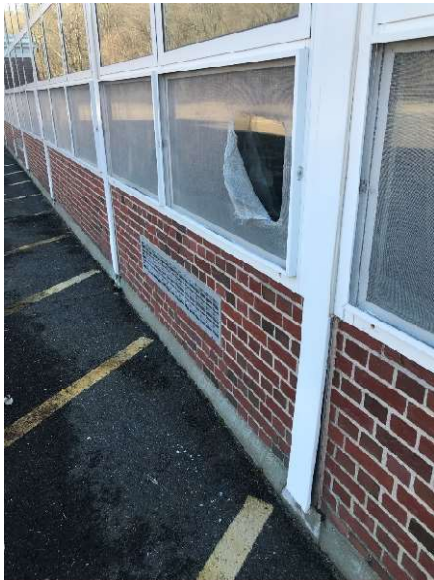
Fig.113 – Damaged insect screen
