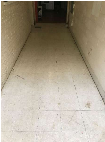
Fig.77 – Damaged vinyl tiles
