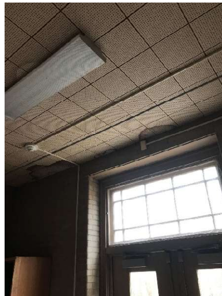
Fig.96 – Damaged ceiling tiles
