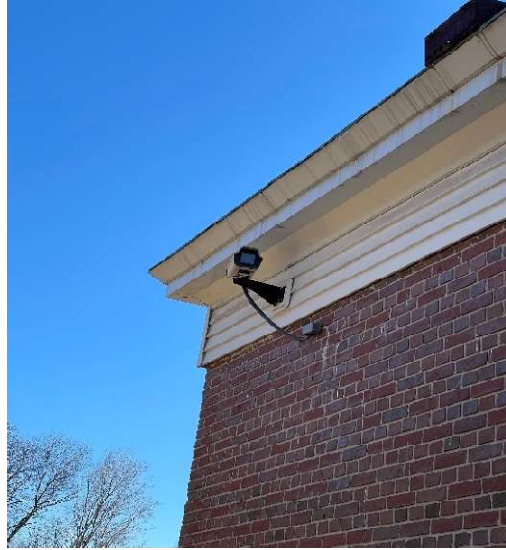
Figure 9: Exterior Wall Mounted Camera.
