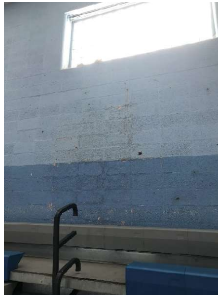
Fig.34 – Signs of water damage on wall
