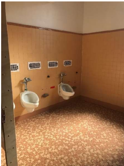
Fig.63– Missing urinal screens
