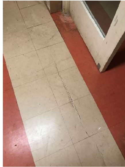
Fig.88 – Damaged vinyl tiles
