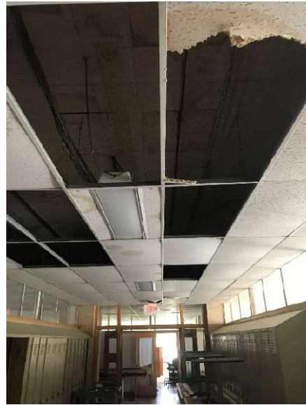
Fig.94 – Damaged ceiling tiles
