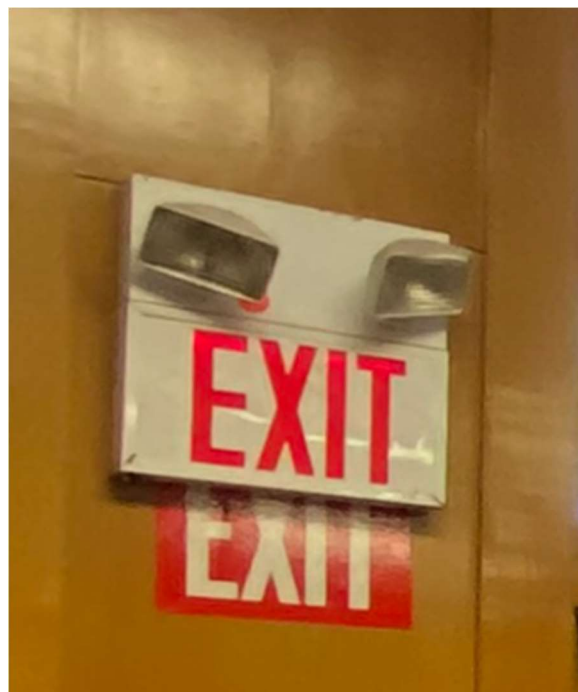
Figure 4: Exit Sign with Emergency Lights.
