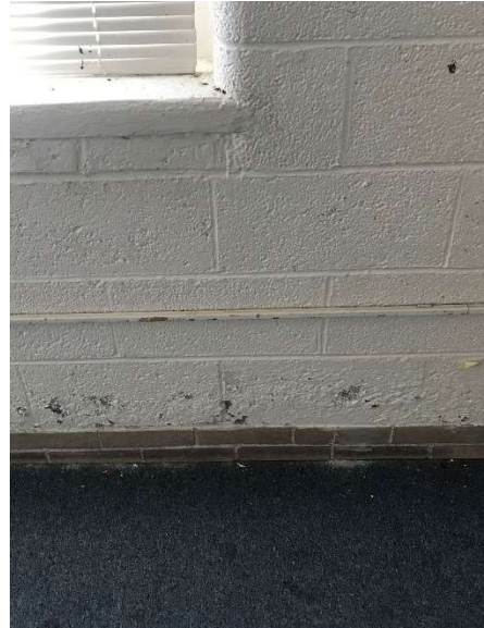
Fig.20 – Damaged CMU Wall
