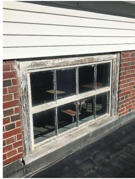
Fig.112 – Damaged window trims
