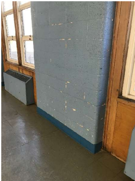
Fig.33 – Damaged wall paint
