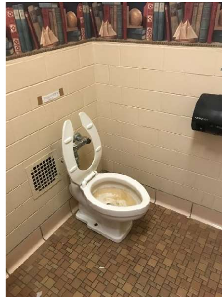
Fig.74 – Grab bars missing
