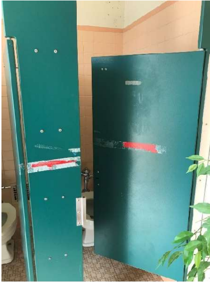
Fig.67– Damaged toilet partitions
