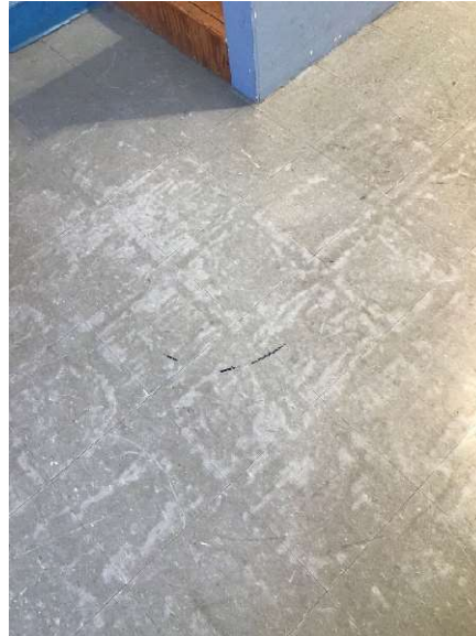
Fig.30 – Damaged VCT floor
