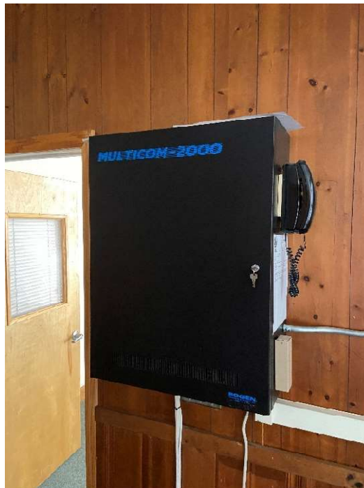
Figure 10: Telephone Control Panel - Bogen Multicom-2000.
