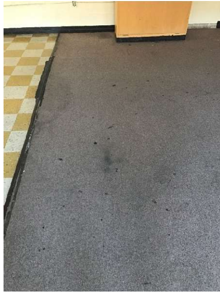
Fig.12 – Stained/Damaged Carpet Floor
