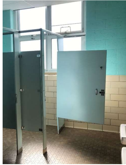
Fig.70 – Damaged ADA stall door
