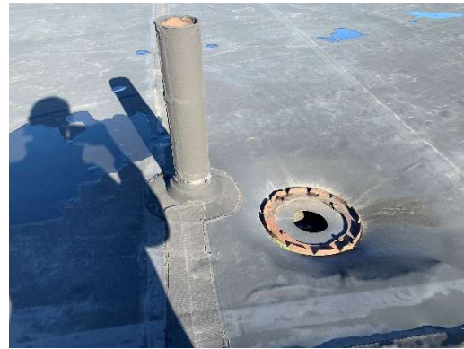
Fig. 8 – Roof drain with missing dome
