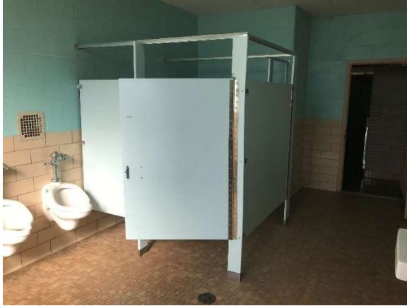
Fig.71– Damaged ADA stall door
