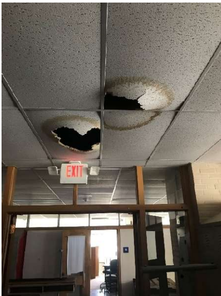
Fig.95 – Damaged ceiling tiles
