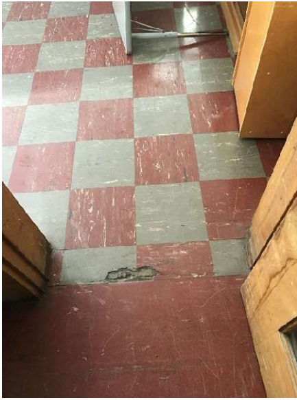
Fig.15 – Damaged VCT Floor
