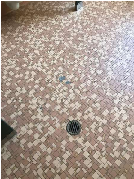
Fig.51 – Damaged ceramic floor
