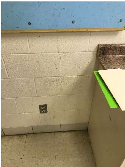
Fig.81 – Cracked CMU wall
