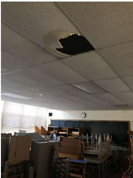
Fig.21 – Damaged ACT tiles
