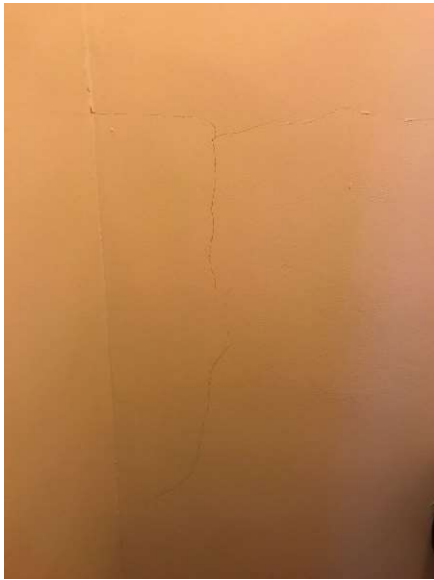
Fig.45 – Cracked GWB wall
