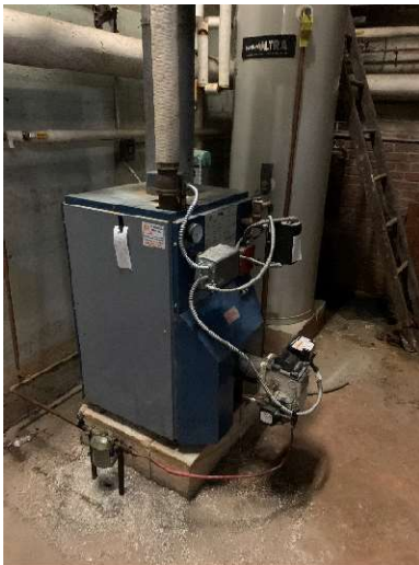
Fig. 6 – Utica Boiler and HPC water heater
