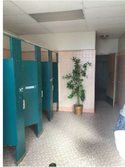
Fig.68 – No ADA toilet stall
