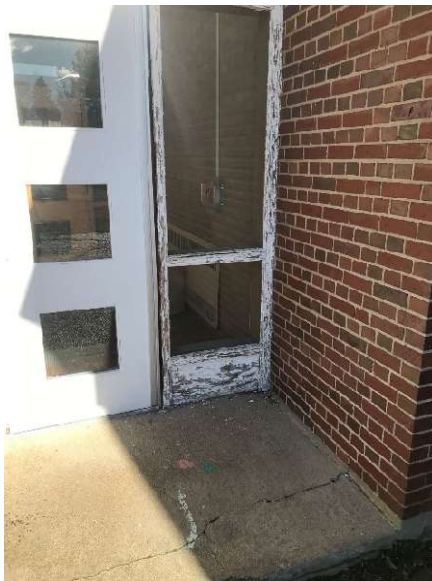
Fig.117 – Damaged door frame
