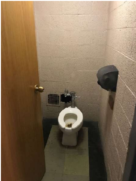
Fig.105 – Damaged CMU wall
