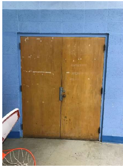
Fig.38 – Damaged wood door
