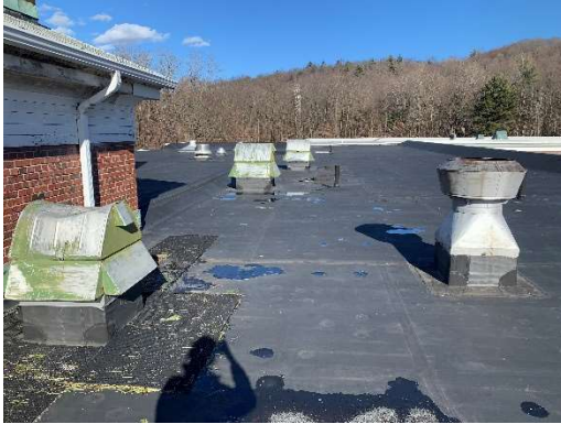
Fig. 12 – Snow hood with snow damage
