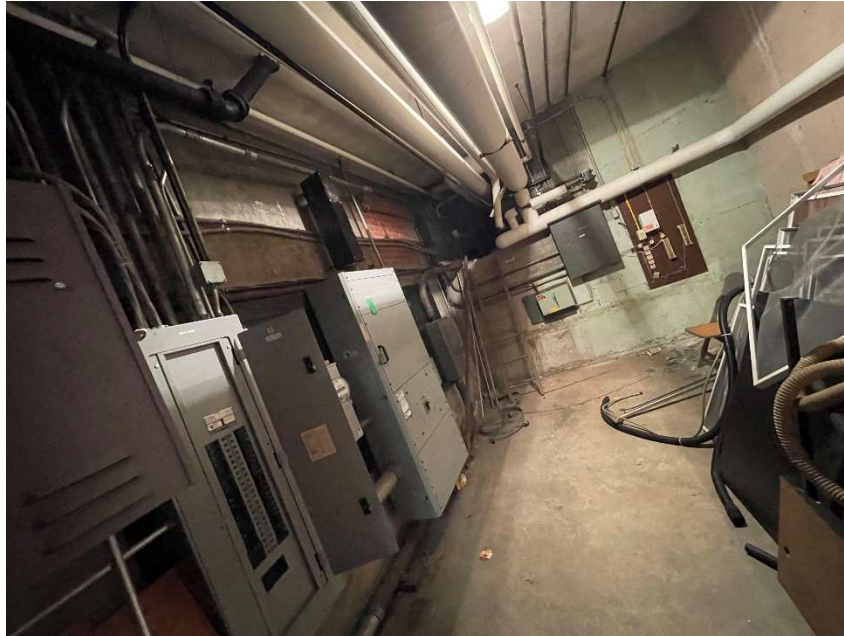
Figure 2: Panel "MDP", Utility Meter, Main Service Disconnect & Old Service Disconnect.
