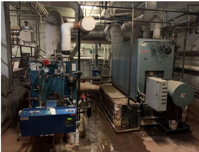
Fig. 1 – Boiler #1 and Boiler #2
