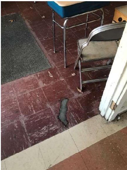
Fig.89 – Damaged vinyl tiles
