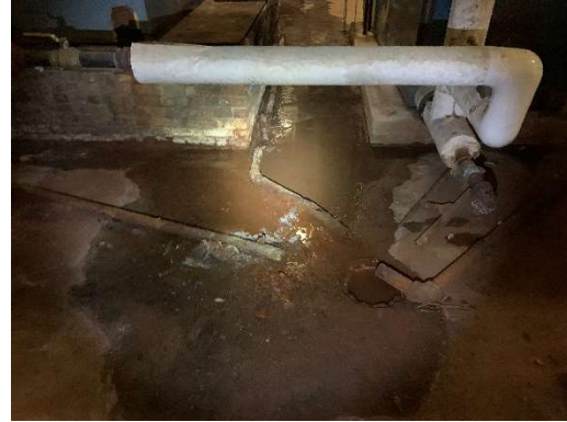
Fig 3. – Failed boiler drain piping
