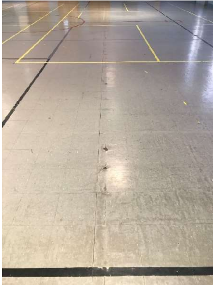
Fig.29 – Damaged VCT floor
