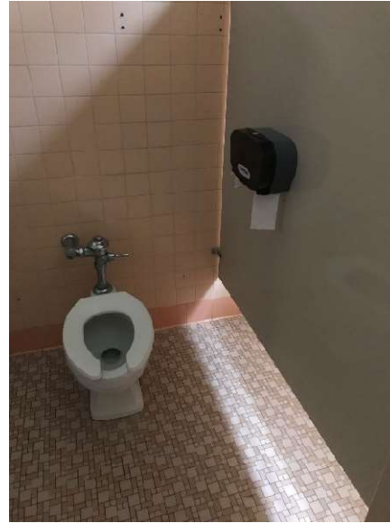
Fig.48 – Damaged wall tile
