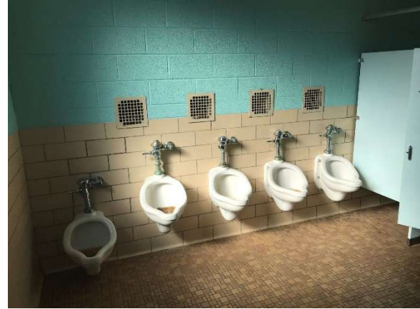
Fig.72 – No urinal screens
