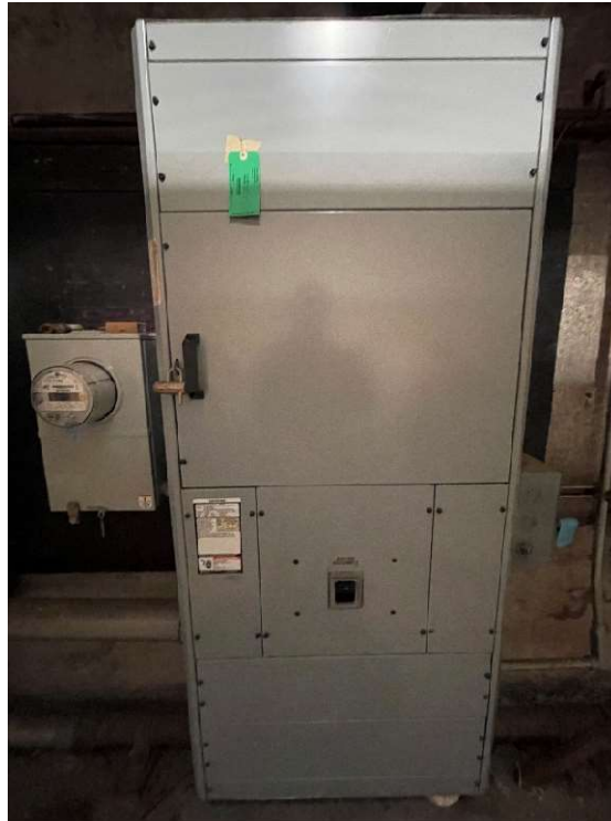
Figure 1: Existing Siemens 600A Service Disconnect.
