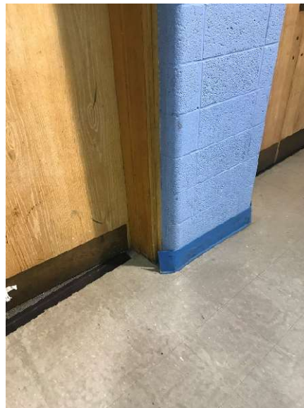
Fig.32 – Loose Vinyl wall base
