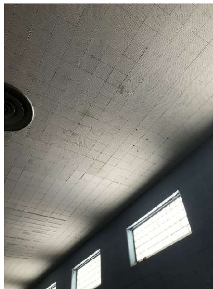
Fig.36 – Stained ceiling tiles
