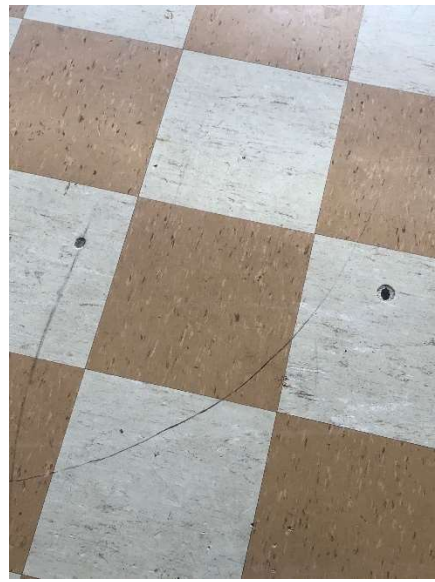
Fig.16 – Damaged VCT Floor
