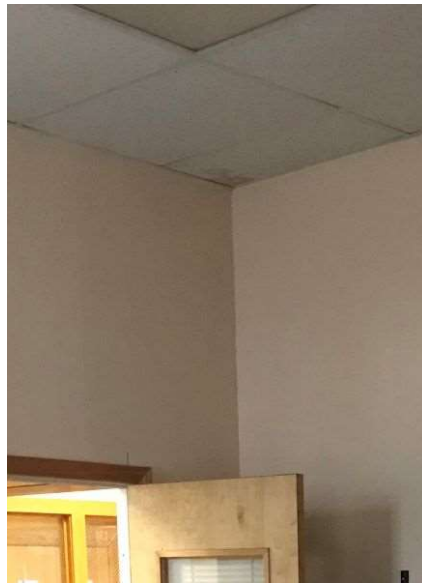
Fig.10 – Damaged ceiling tile
