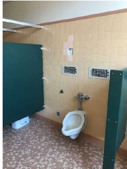
Fig.52 – Damaged ceramic wall
