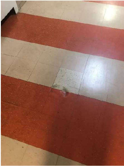
Fig.87 – Damaged vinyl tiles
