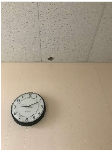
Fig.9 – Damaged ceiling tile
