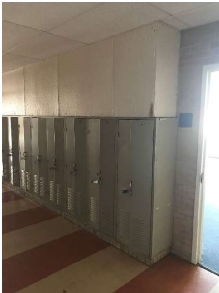
Fig.91 – Damaged wall boards
