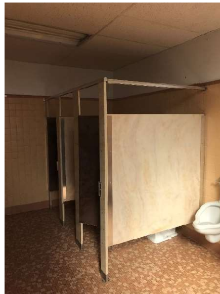
Fig.64 – Missing toilet stall door
