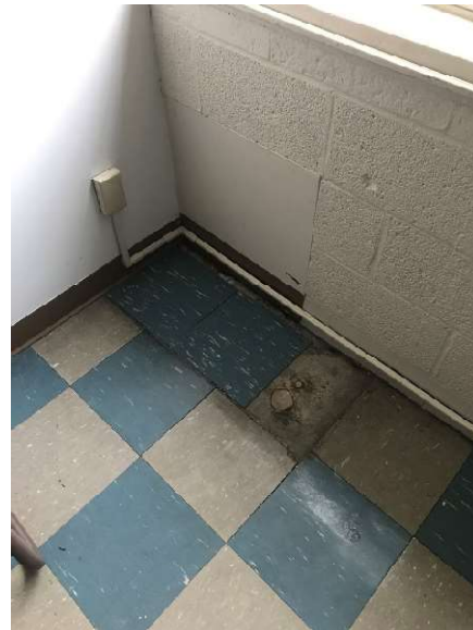
Fig.14 – Damaged VCT Floor
