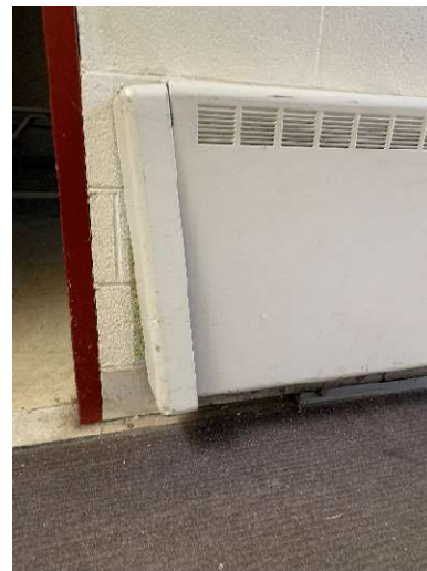
Fig. 11 – Convector with damaged cover
