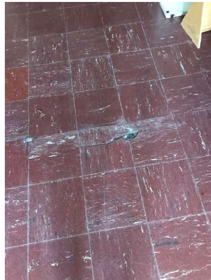
Fig.90 – Damaged vinyl tiles
