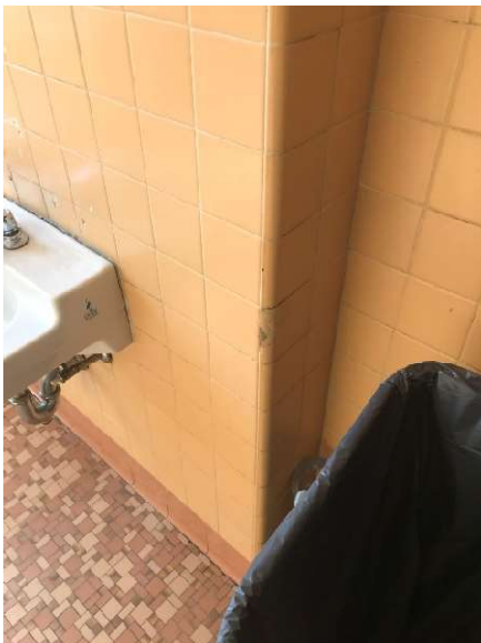
Fig.59– Damaged ceramic wall
