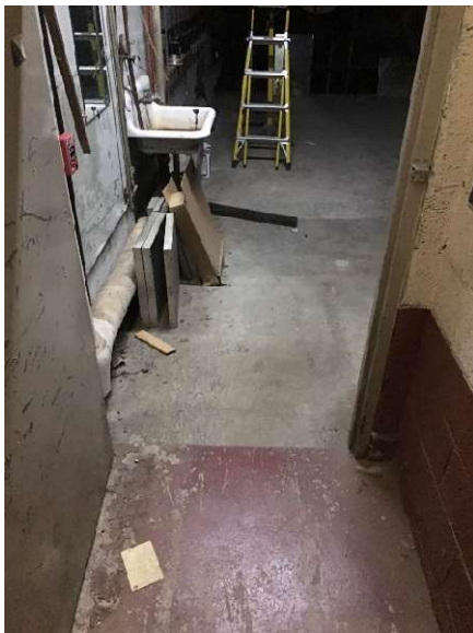
Fig.1 – Damaged floor coating
