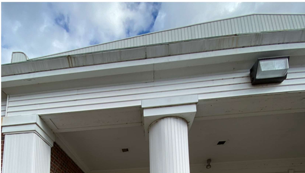
Figure 7: Exterior Wall Pack and Recessed Fixtures.
