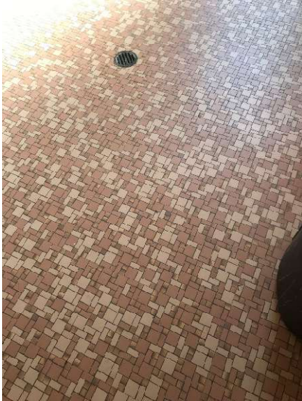
Fig.57– Damaged ceramic floor
