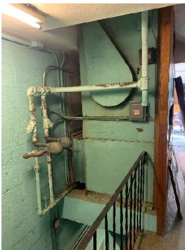
Fig. 13 – Supply fan with steam coil
