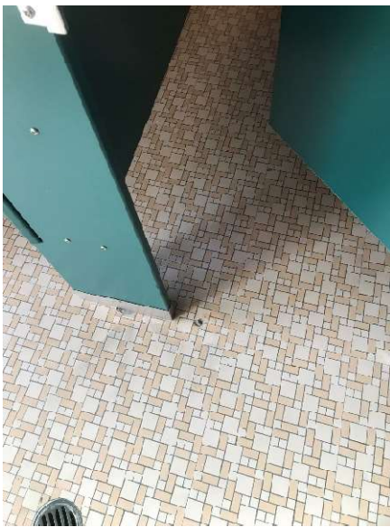
Fig.65– Damaged ceramic floor
