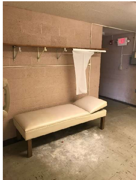
Fig.102 – Damaged Vinyl floor tiles
