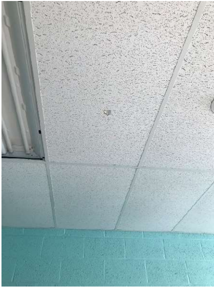
Fig.69– Damaged ACT tile
