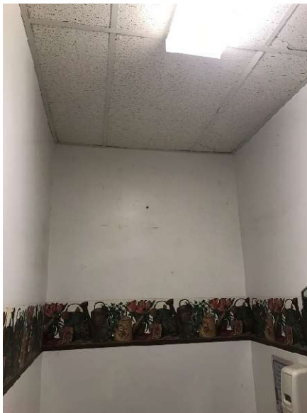
Fig.75 – Damaged wall & ceiling tiles
