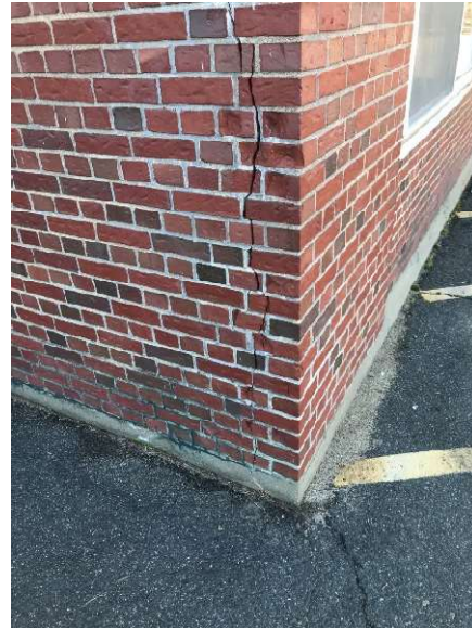
Fig.110 – Cracked brick veneer/foundation wall
