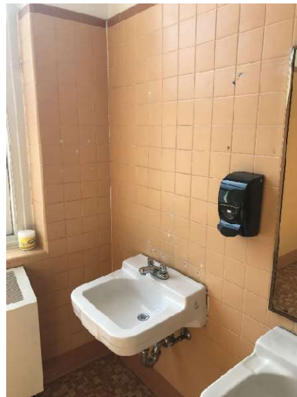
Fig.60 – Damaged ceramic wall
