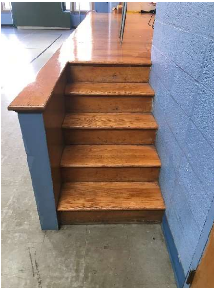
Fig.43 – No ADA handrails at stairs
