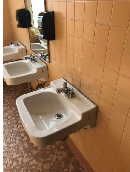
Fig.58 – Damaged ceramic wall
