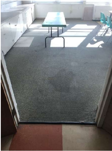
Fig.11 – Stained/Damaged Carpet Floor
