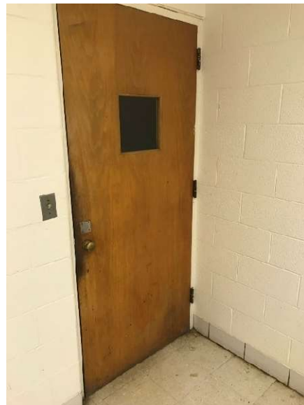
Fig.82 – Worn door and hardware
