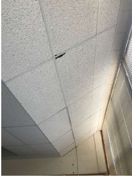
Fig.23 – Damaged ACT tiles
