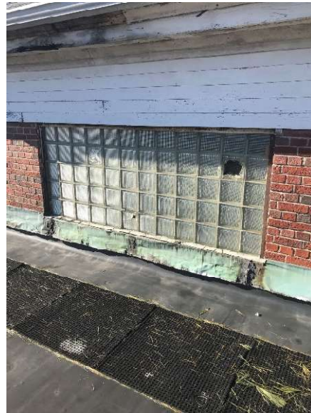
Fig.114 – Damaged glass block window
