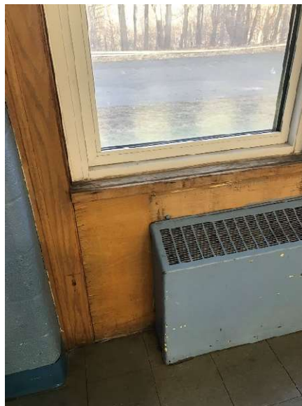
Fig.40 – Damaged wood panels/trims
