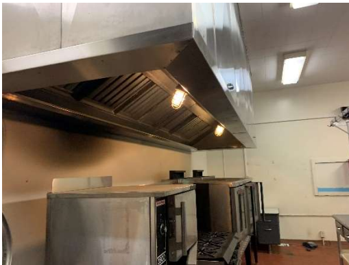
Fig. 14 – Hood serving cooking equipment
