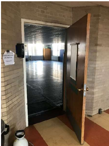
Fig.85 – Worn door hardware
