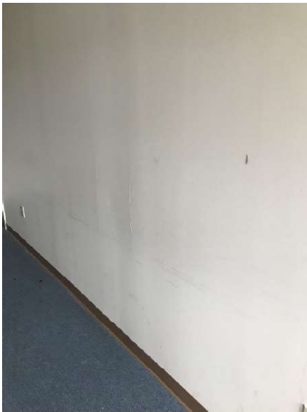
Fig.17 – Damaged GWB wall
