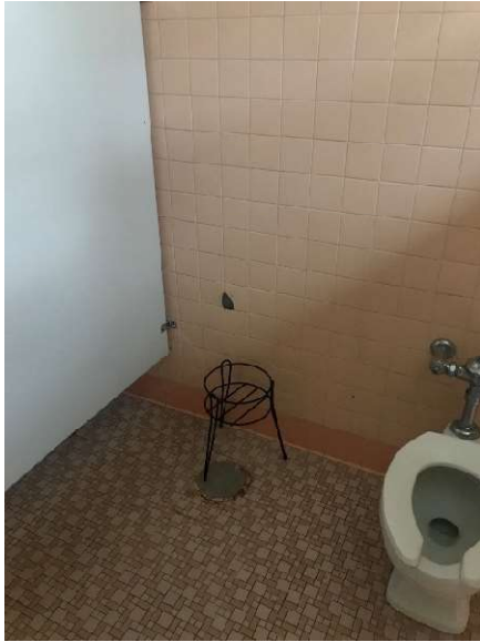
Fig.47 – Damaged ceramic floor & wall tile
