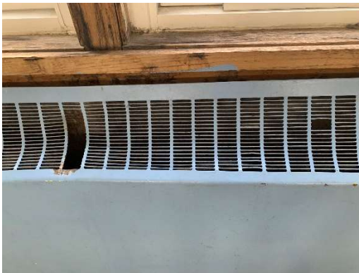
Fig. 10 – Unit ventilator with damaged grille
