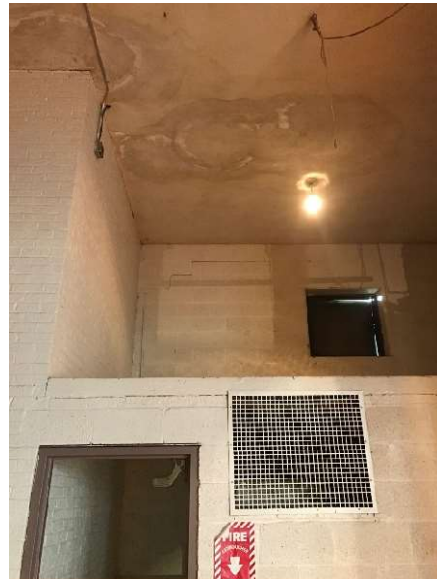
Fig.42 – Water damage stains
