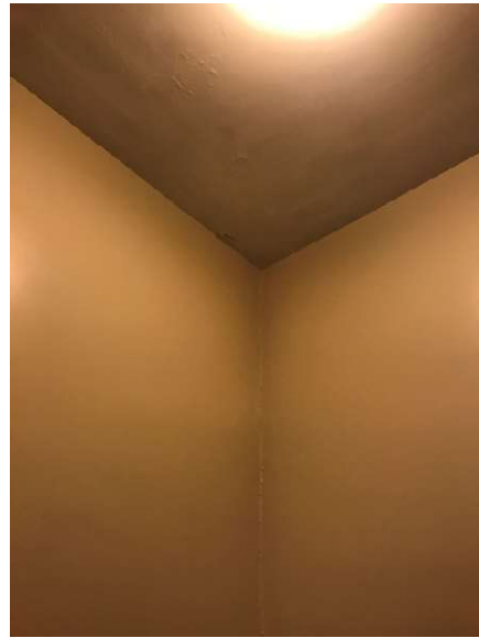
Fig.46 – Damaged GWB ceiling
