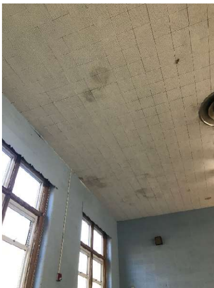
Fig.35 – Stained ceiling tiles
