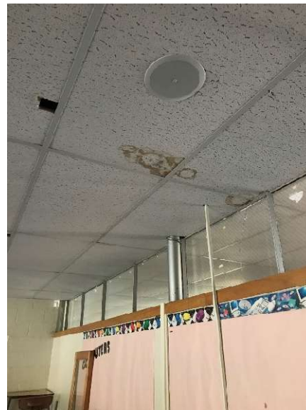
Fig.22 – Damaged ACT tiles
