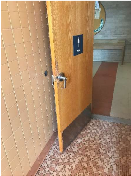
Fig.61– Damaged wood door and hardware
