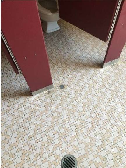
Fig.55– Damaged ceramic floor
