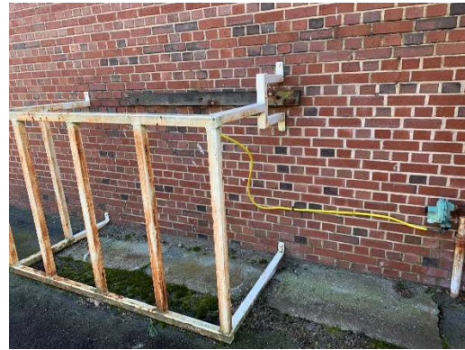
Fig. 18 – NG meter and tank location
