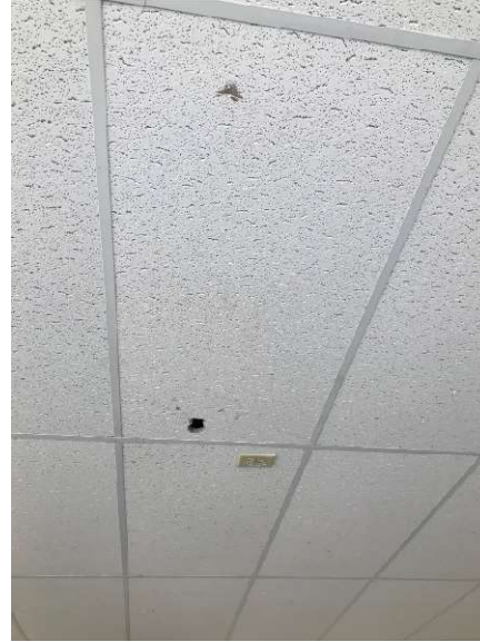
Fig.24 – Damaged ACT tiles
