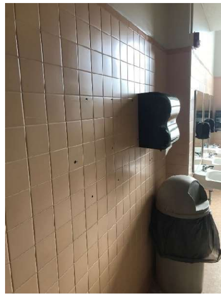
Fig.66 – Damaged ceramic wall
