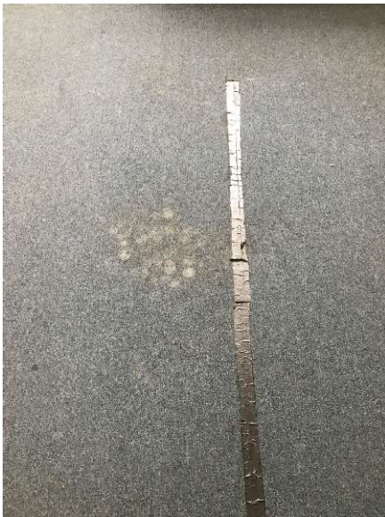
Fig.13 – Damaged Carpet Floor
