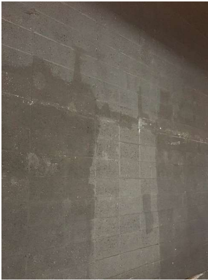
Fig.41 – Stage rear wall paint color mismatch
