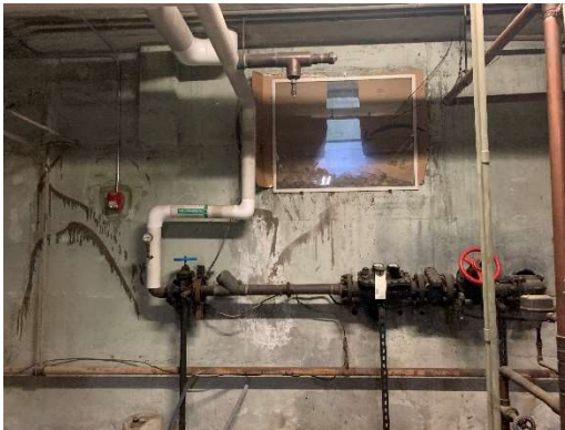
Fig. 5 – Water service entrance
