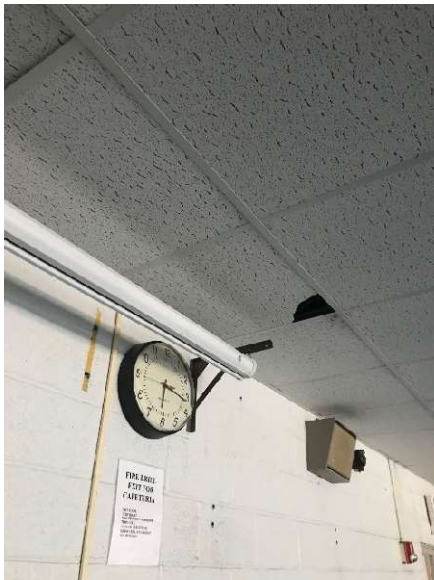
Fig.83 – Damaged ACT tile
