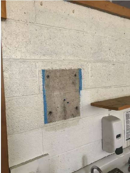
Fig.19 – Damaged CMU wall
