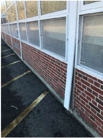
Fig.111 – Damaged/loose window trim
