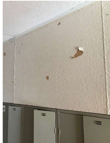
Fig.92 – Damaged wall boards
