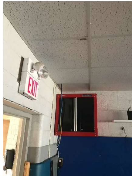
Fig.84 – Damaged ACT tile
