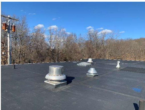
Fig. 16 – Exhaust fans serving kitchen hoods
