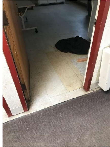
Fig.80 – Damaged vinyl tiles
