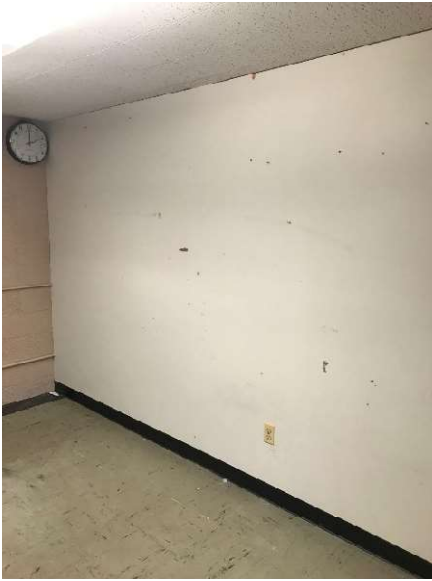
Fig.103 – Damaged GWB wall
